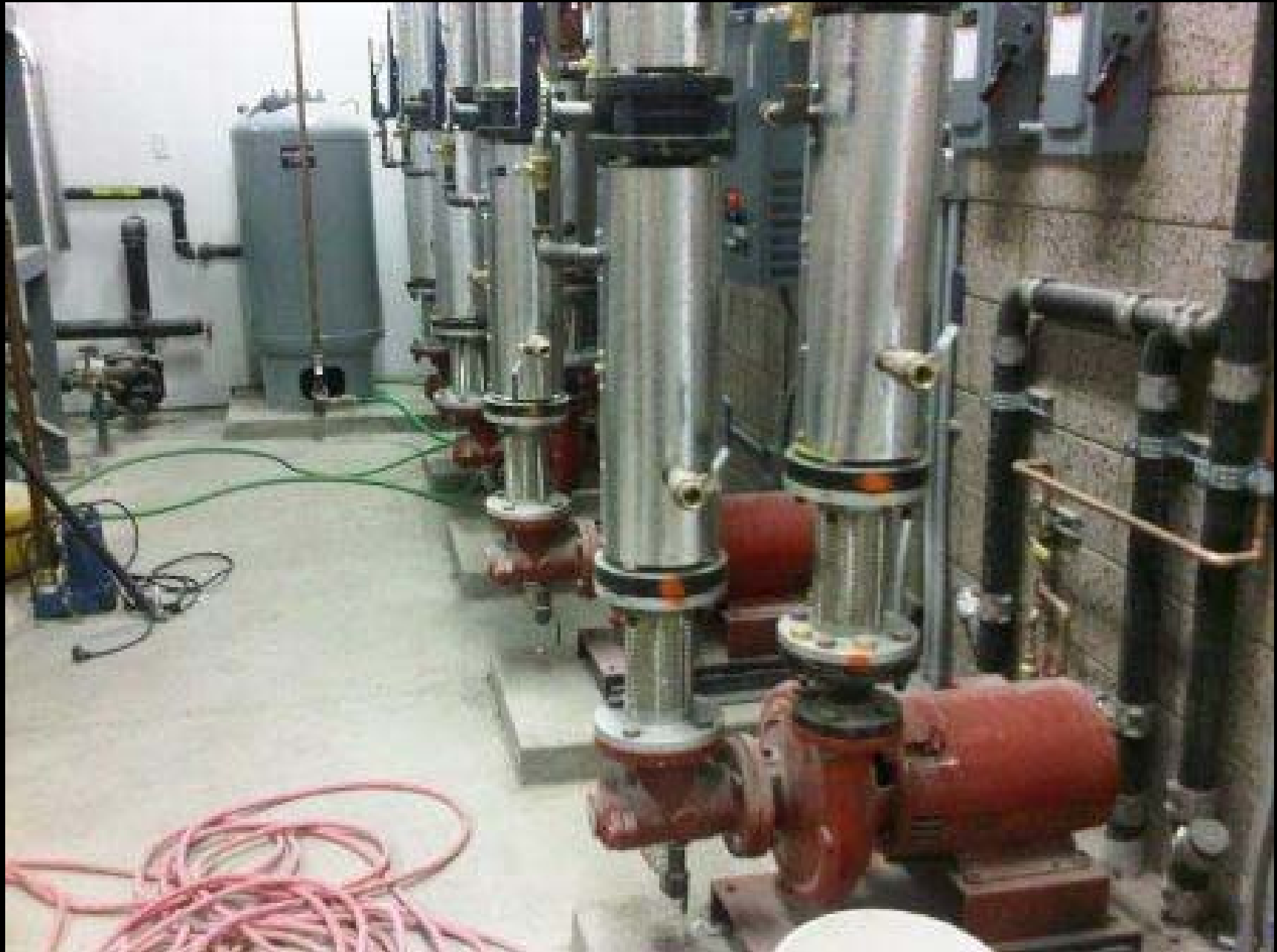
3/15/10 – CTE Mechanical Room
